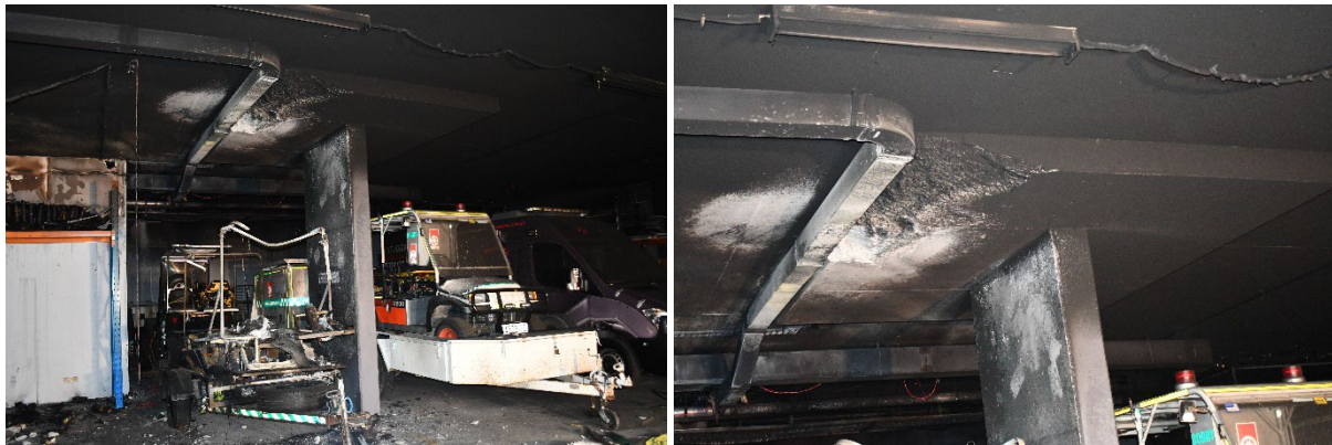
FIGURE 15 PHOTOS SHOWING CONCRETE SPALLING ABOVE THE FIRE AFFECTED GOLF CART, WHICH CAUGHT FIRE IN BURWOOD, NSW IN SEPTEMBER 2023
